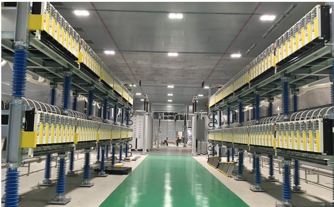
The Stafford Centre for Excellence for HVDC test facility.
